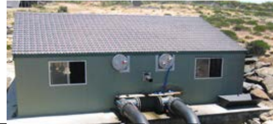
Drinking water pumping station
